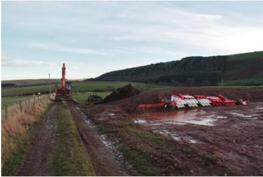
Construction work begins on our wind turbine at Hoprigshiels in Scottish Borders
