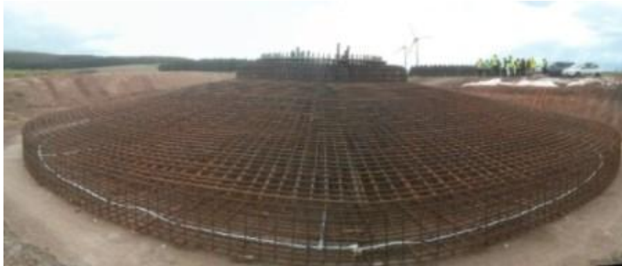
Foundation reinforcement cage - the bright metal strip is part of the earthing cabling for lightning conductor.
